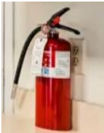
FIRE EXTINGUISHER – located in the kitchen
